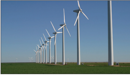
Fig. 5. Wind power plant
