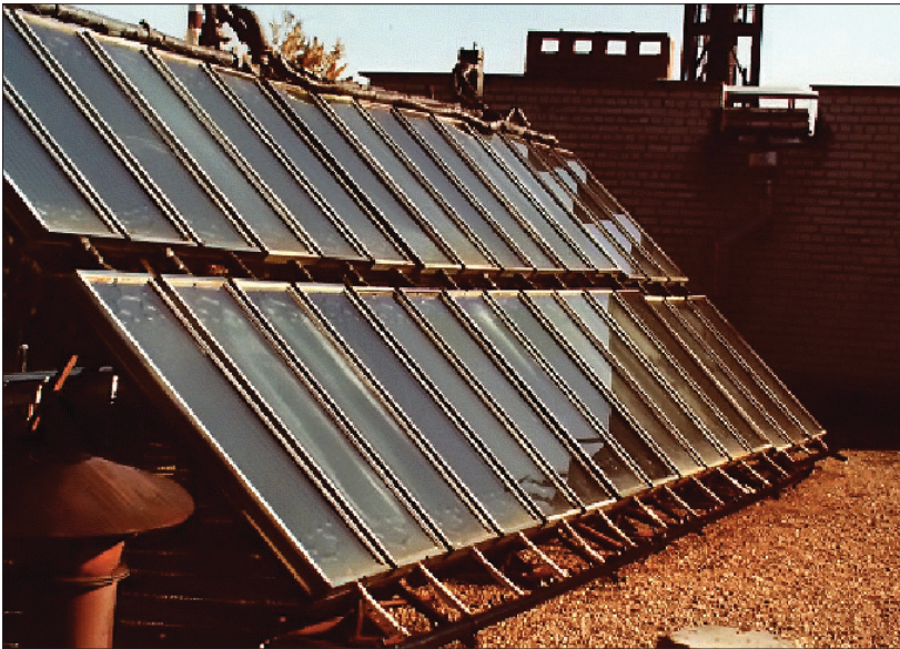
Figure 3. Experimental module of solar heating system
