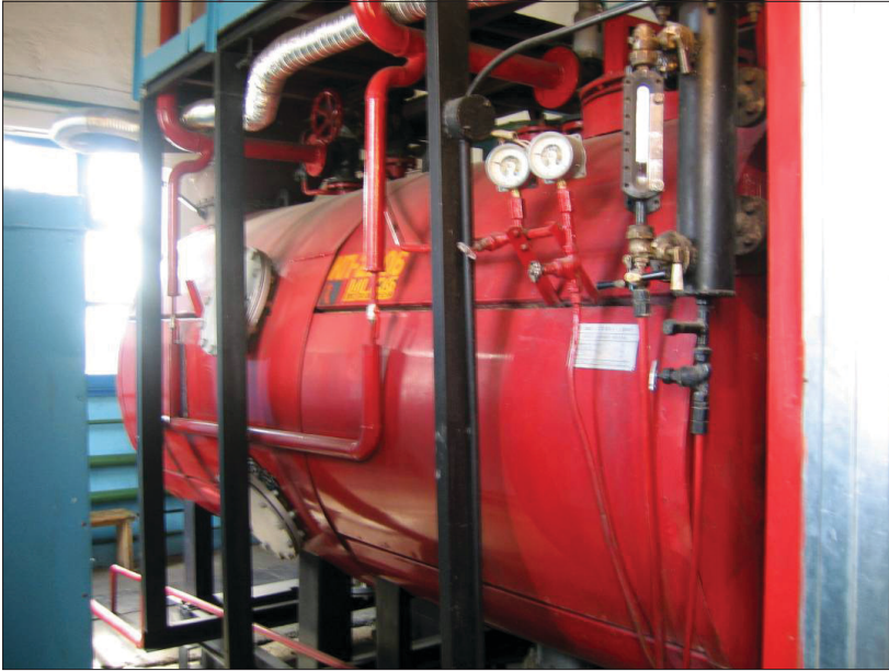
Figure 4. Boiler with capacity of 1.2 MW
