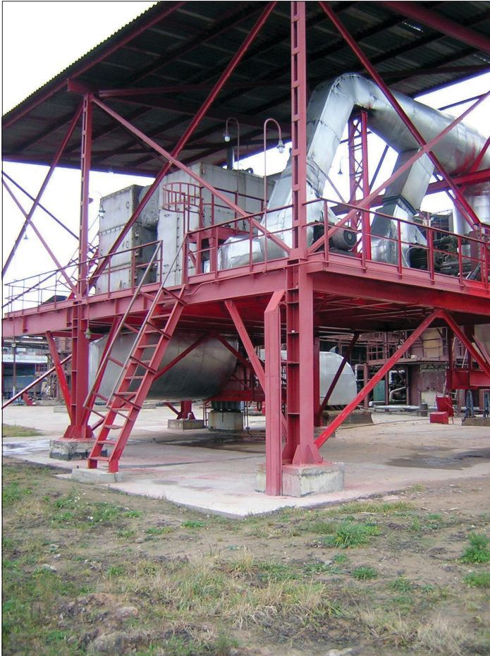
Figure 5. Picture of the salvage heat exchanger with output of 10 t/h of steam
